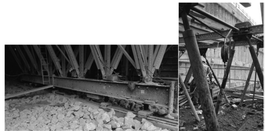
Figure 6. Union of the Bogie system assemblies Pre-assembly of the vault (Source: Author).
